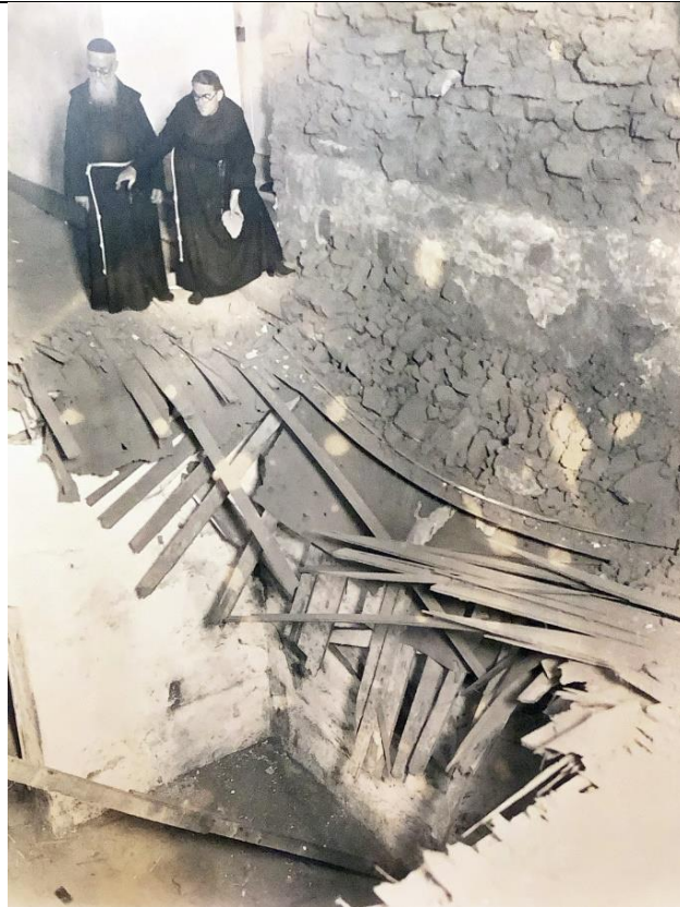
Figure 23. View of the floor collapse where Father Augustine and Brother Odoric had fallen through the floor. Photo credit: Santa Barbara Historical Museum, Gledhill Library.
